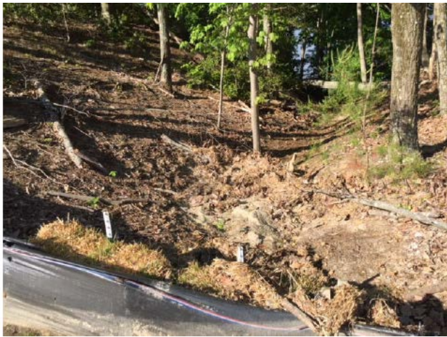
Exhibit 5: Photo (Figure 8) from May 8, 2018 DEQ inspection report
