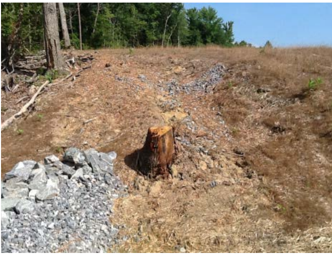
Exhibit 7: Photo (Figure 6) of the July 13, 2018 DEQ inspection report of Virginia True property. Note the inadequate soil stabilization on a steep slope at edge of cleared area (more than 7 months after the Stop Work Order issued by Richmond County.)
